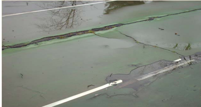
Example of wear and tear on city's hard-surface courts
