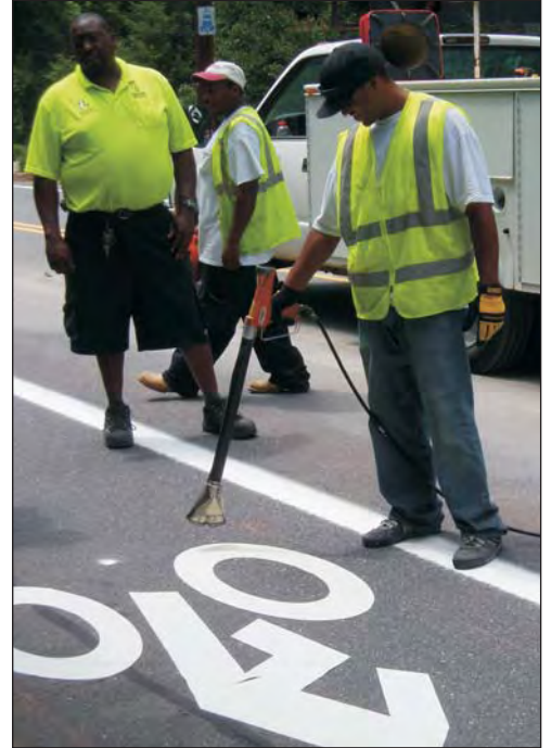
Winston-Salem DOT crews installing the heat activated stencils in the first bike lane on Reynolda Road.
