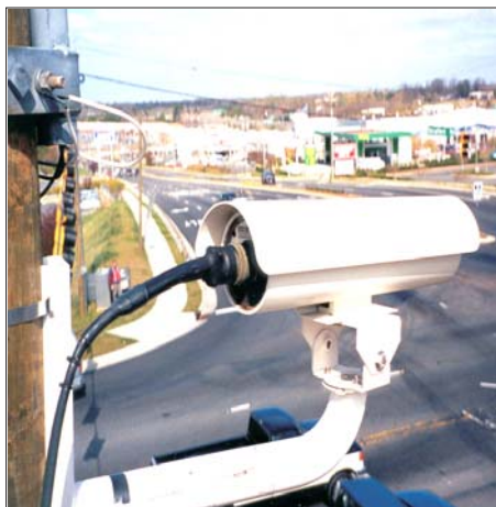
Video traffic monitoring at Hanes Mall Blvd. and S. Stratford Rd.
