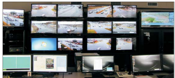
Traffic Signal System Monitoring Video Wall.
